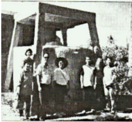
Water Resource Assessment group in front of partly finished water tank in Barrio Ipil (Boac). Above are L to R, two government social workers, Dave & Macrine, two CFO Rep. and taller person is Pablito Alarcon from the Feed The Hungry group of Washington, DC.
